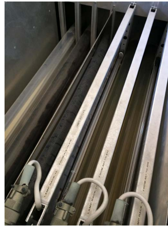
Water gets pumped from the tertiary pond at 15 litres per second through the UV system
