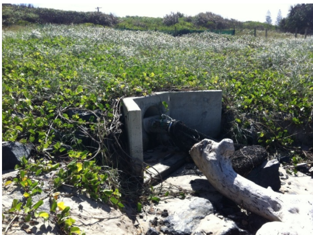
Photo 5: Outlets in inaccessible areas are difficult to access and not regularly maintained (Lennox beach headland)
