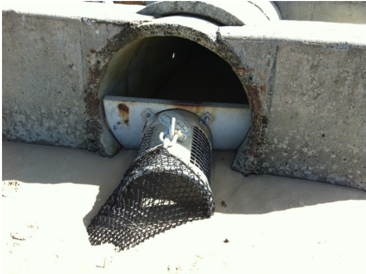
Photo 12: Sock installed on stormwater pipe discharging onto Seven Mile Beach, Lennox Head
