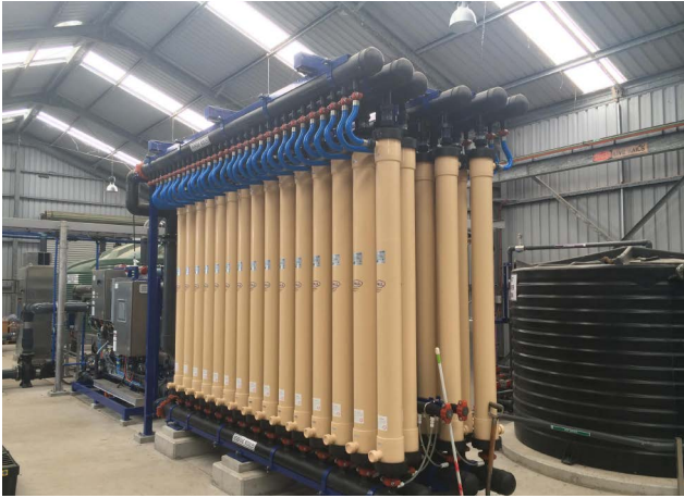
Water intended for re-use is past through these membrane filters which further clean the water.
