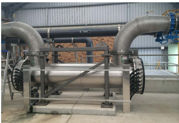
UV disinfection gets rid of any unwanted pathogens. It allows 40 litres of water to pass through it per second.
