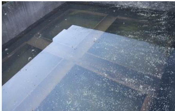
INSIDE FILTRATION TANK
