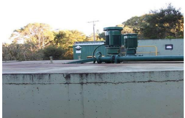
CLEAR WATER TANK & CLEAR WATER PUMPS
