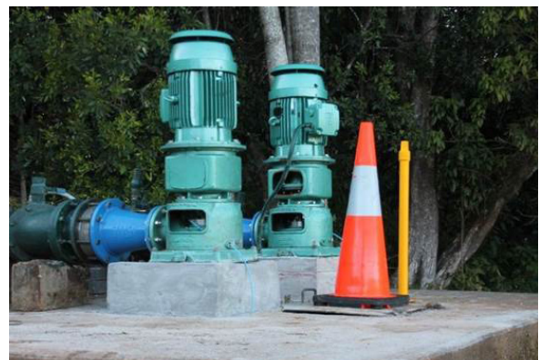
RAW WATER PUMPS
