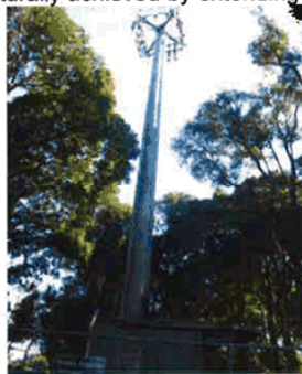
Figure 1 – Existing Telstra facility
