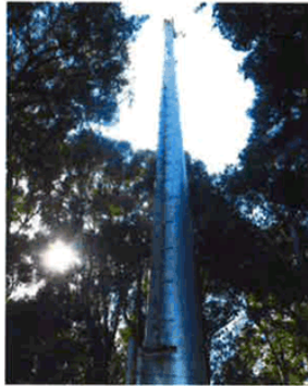
Figure 2 – Existing Optus facility
