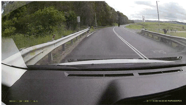
Ross Lane – Westbound gap in guard rail for property access west of North Creek.
