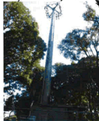
Figure 1 – Existing Telstra facility
