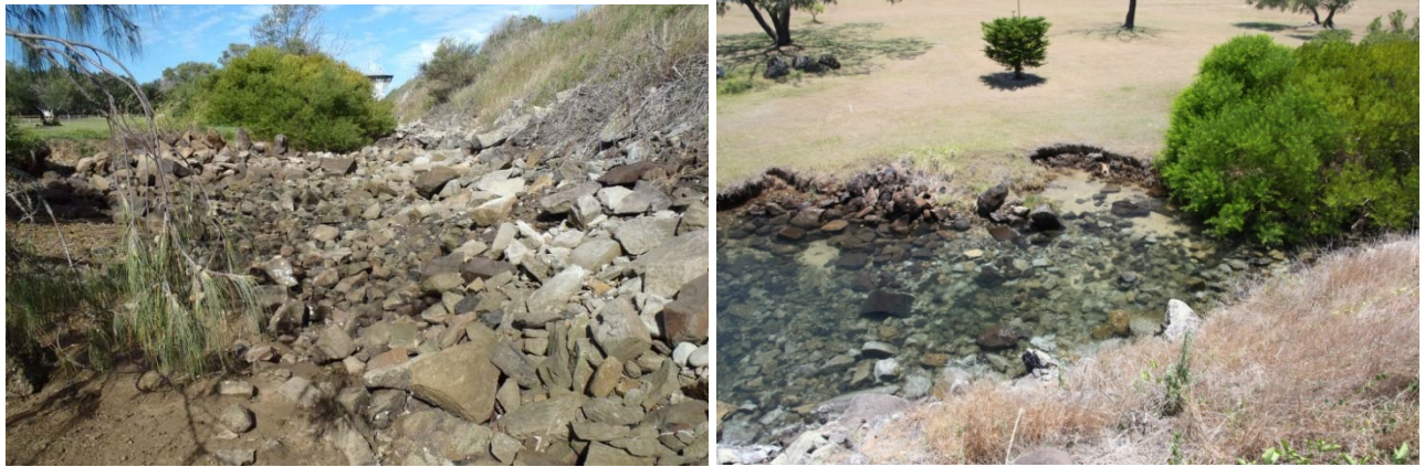
Figure 17: Continued erosion at the eastern extremity of the East Arm
