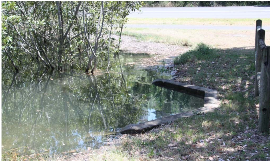
Figure 19: Tidal inundation of stormwater drain (January 2014)
