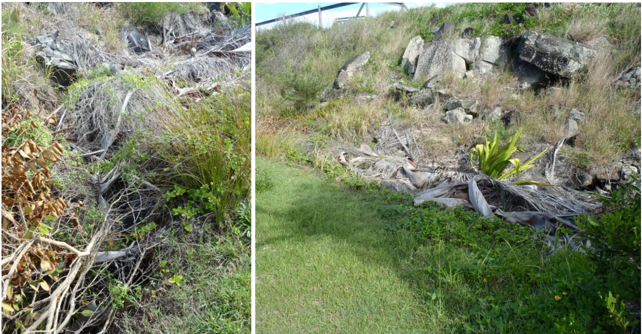
Figure 16: Sink holes along the training wall partially covered by garden clippings
