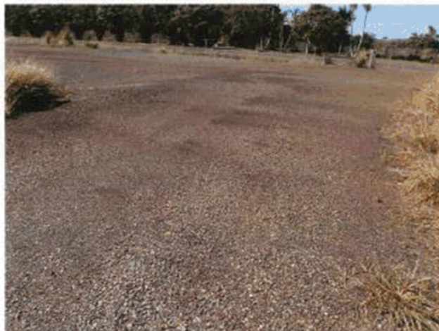
Plate 6: General view of asphalt area showing oil staining from vehicles
