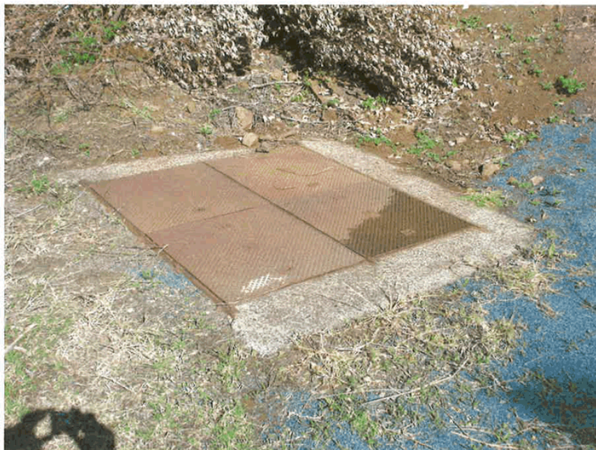
Photo 4. Storm Water Access Pit Cover Top Lot 1.
