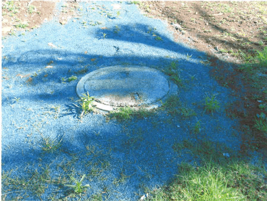
Photo 5. Storm Water Access Pit Cover Top Lot 1.
