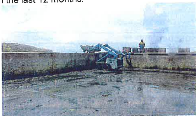
POOL FLOOR SLUMPED 80 MM ALONG CRACK
