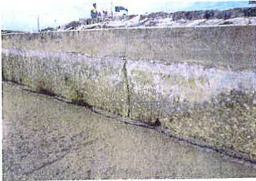
CRACKS IN THE POOL
