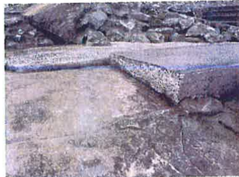
BROKEN ACCESS PATH
