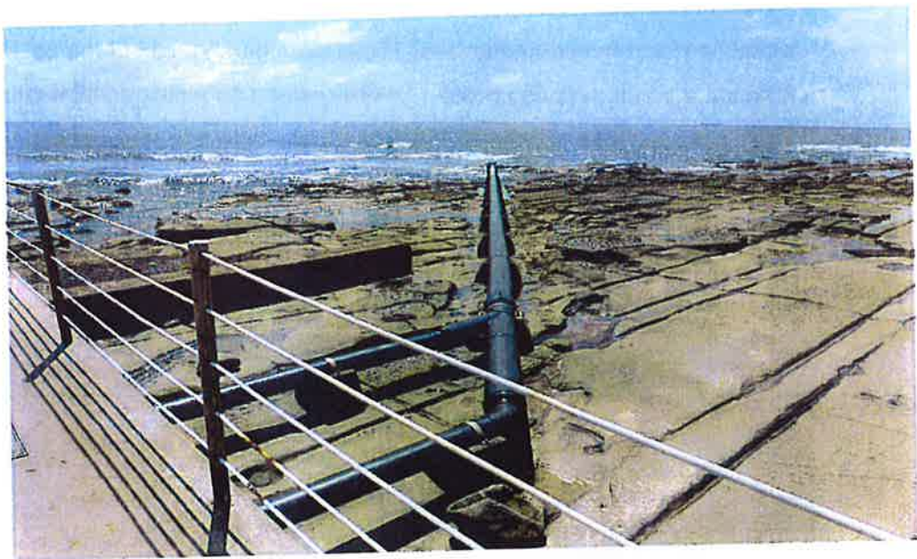
Dry Mounted pump inlet pipe (Entrance Ocean baths)
