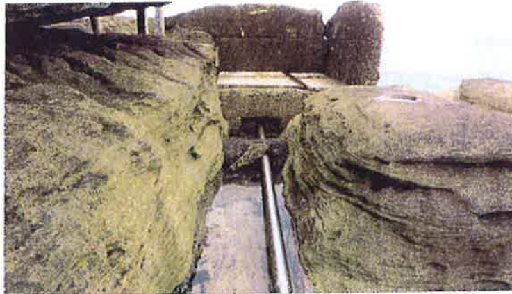
PUMP HOUSE & STAINLESS STEEL INLET PIPE
