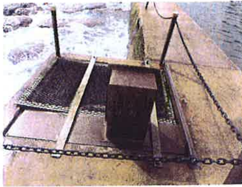
PUMP & PUMP INLET
