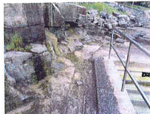
POOL DECK SLIP TRIP HAZARDS
