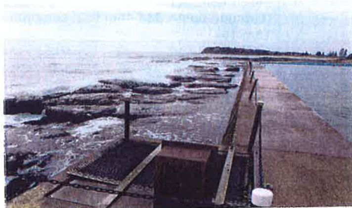
ROCK SHELF WITH PUMP & PUMP INLET (FOREGROUND)
