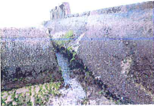
UNDERMINED POOL WALL
