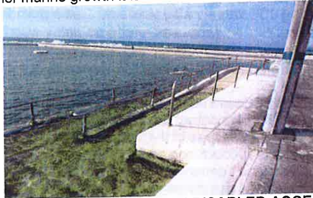
STAINLESS STEEL USED IN DISABLED ACCESS
