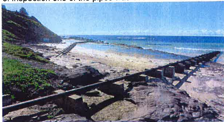
THE TWO INLET PIPES
