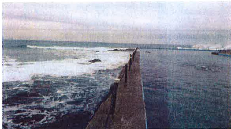
NORTH WALL TO BE REPLACED 2010
