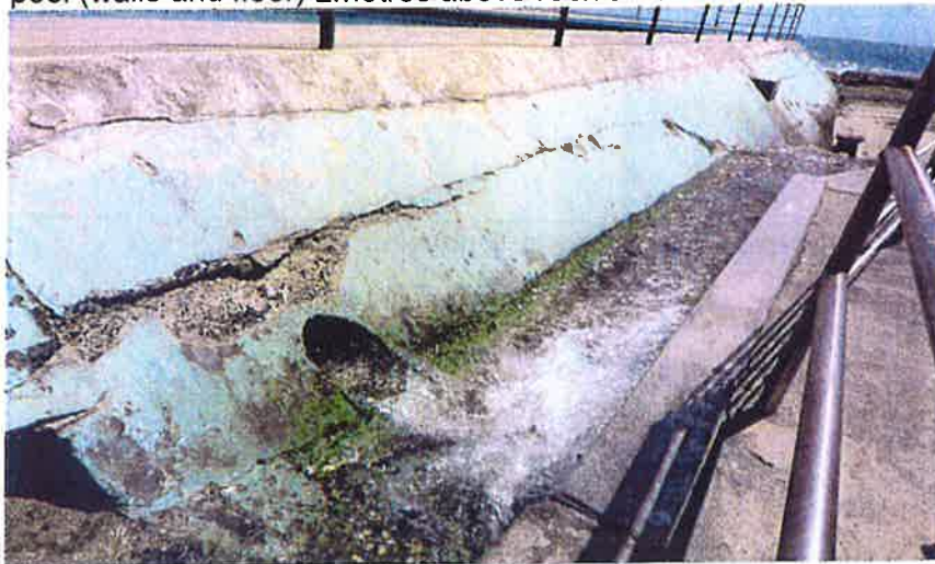
2 METRE POOL WALL NOTE THE CRACK ABOVE DRAIN THIS IS WAS THE OLD POOL HEIGHT BEFOR UPGRADE
