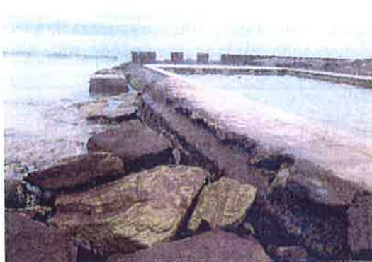
DAMAGED NORTH WALL
