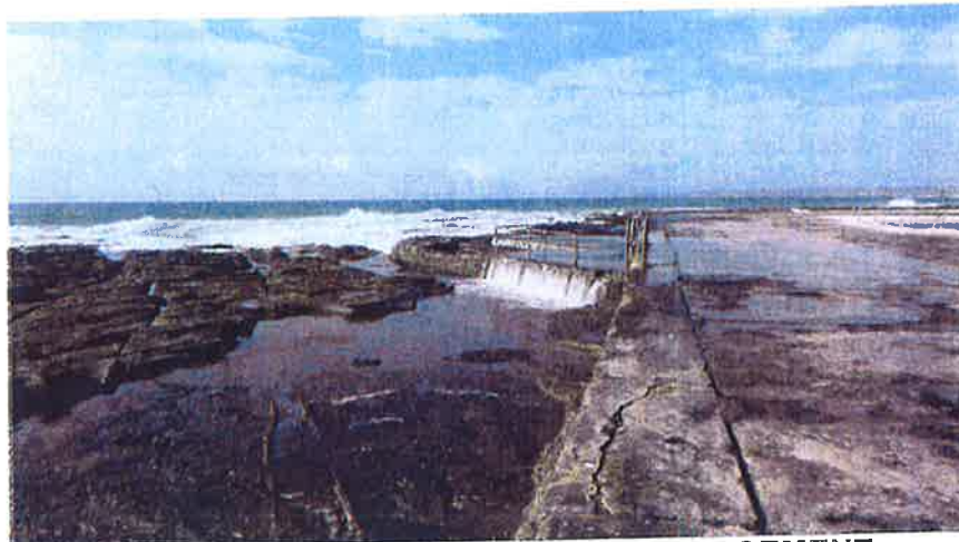
PROMENADE SCHEDULED FOR REPLACEMENT
