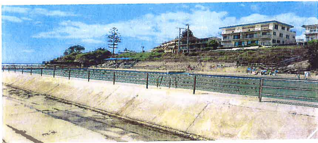
Entrance Ocean baths recent renovations included raising of the pool and surrounds by 600 mm
