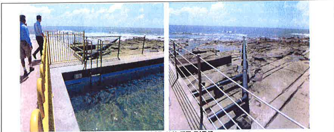
PUMP INLET PIPE
