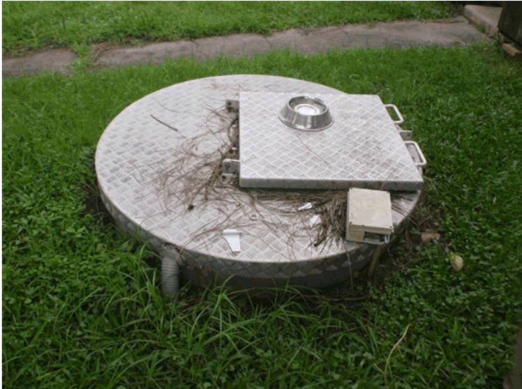
Plate B3: In-ground tank thought to be private sewer pump station.
