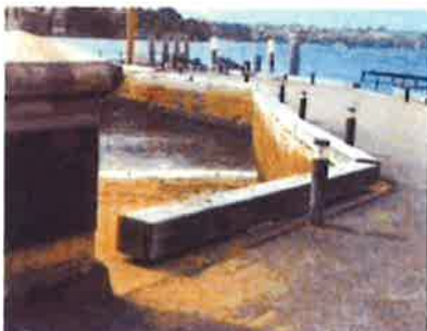
Man of War Steps, Bennelong Point [not recommended as light post and timber corner hazards]
