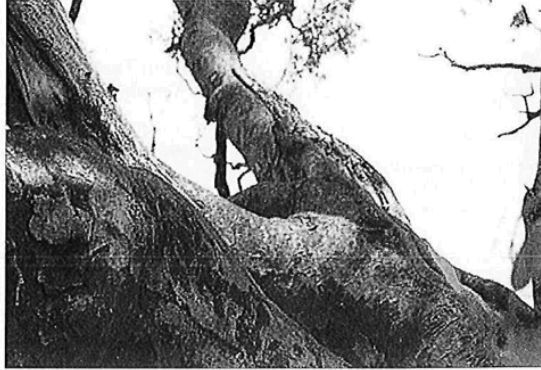
Plate 3 Sunburn and decay on the tops of 3 major branches
