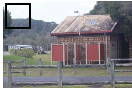
'tired' looking toilet facilities
