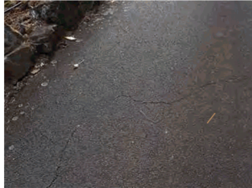
Photo 6. Minor cracks in the bitumen.
