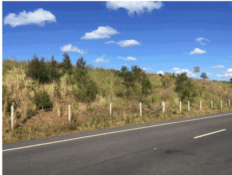
Plate 4: T2E rainforest batter depicted in Plate 3, as at 1 July 2016. Note: Plant growth along the batter is poor with a large number of plant losses.
