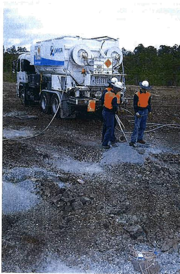
Figure 4 – Blasthole loading at a quarry with a Mobile Manufacturing Unit (MMU). The MMU can accurately measure and deliver the required designed amount and type of explosives into each blasthole.
