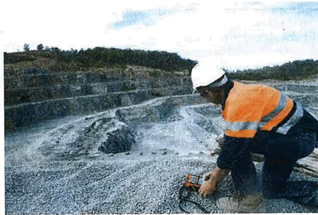
Figure 5 – Shotfirer firing a blast using electronically programmed detonators to ensure vibration and airblast effects from blast are reduced as much as possible.
