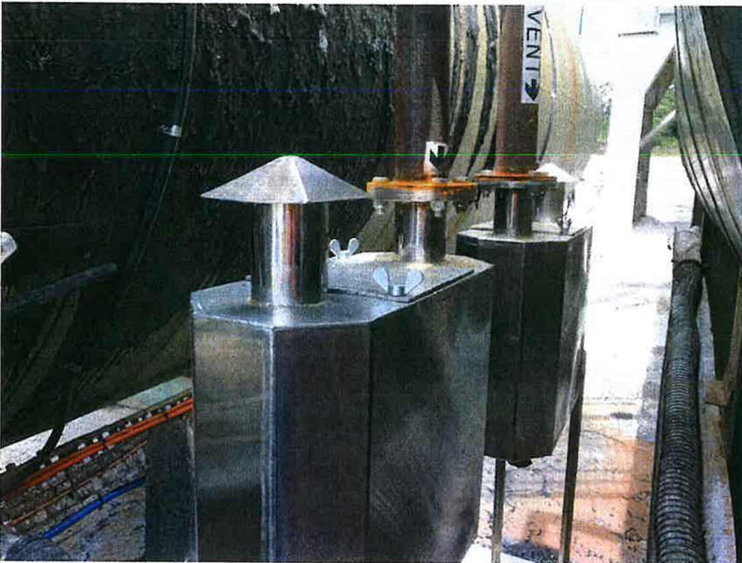
Figure 3-3 Bitumen tanks (above) and carbon filtration units and vents (below) situated between the tanks
