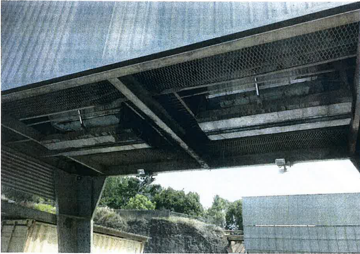
Figure 3-7 Truck asphalt loading facility under the hot asphalt storage bins
