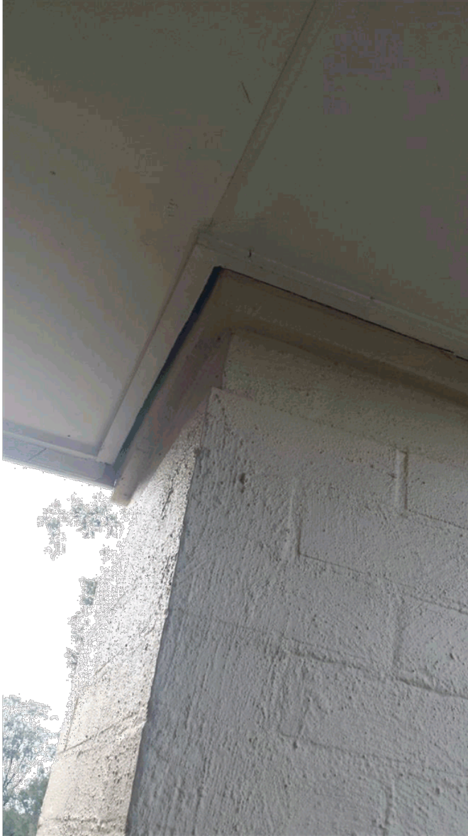
Photo No. 1 – Leaning brick pillar at the entry to the house.
