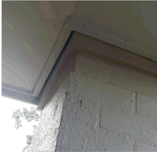
Photo No. 1 – Leaning brick pillar at the entry to the house as photographed on 6 April 2017.
