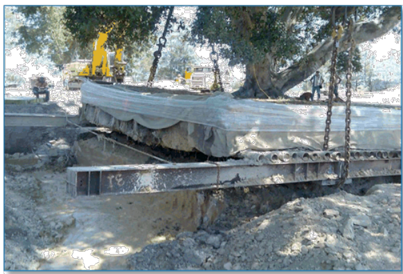
Figure 15. Lifting a very large Ficus microcarpa var 'Hillii' using a pipe raft, under beams and heavy lift cranes.
