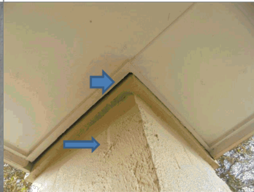
10: Portico column slight rotation and soffit gap
