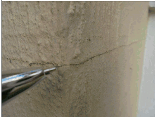
11: Portico column crack
