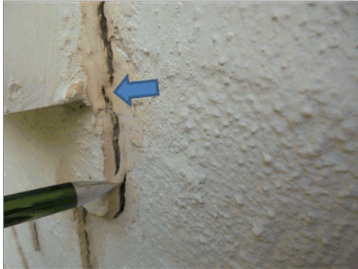
07: Bedroom 2 east wall crack. Note lateral displacement
