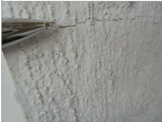
09: Bed 2 crack in south wall
