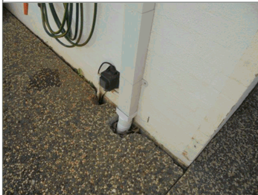
21: The owner found tree roots between the house where the path is lifting at the western side of the office
