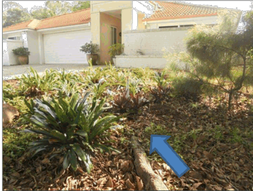
19: Tree roots running towards the house
