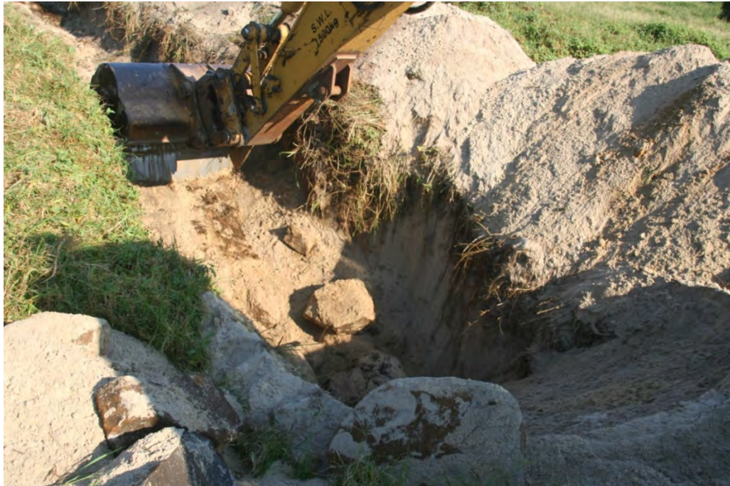
Figure 4-10 Toe Rocks Exposed
