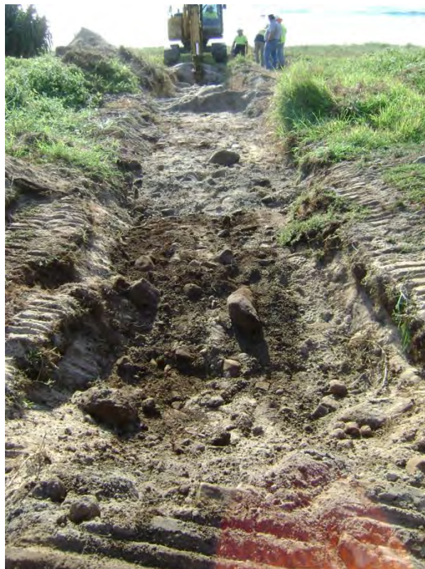
Figure 6: Rock exposure visible following the second excavation on 10 th October, adjacent to Line 18.
