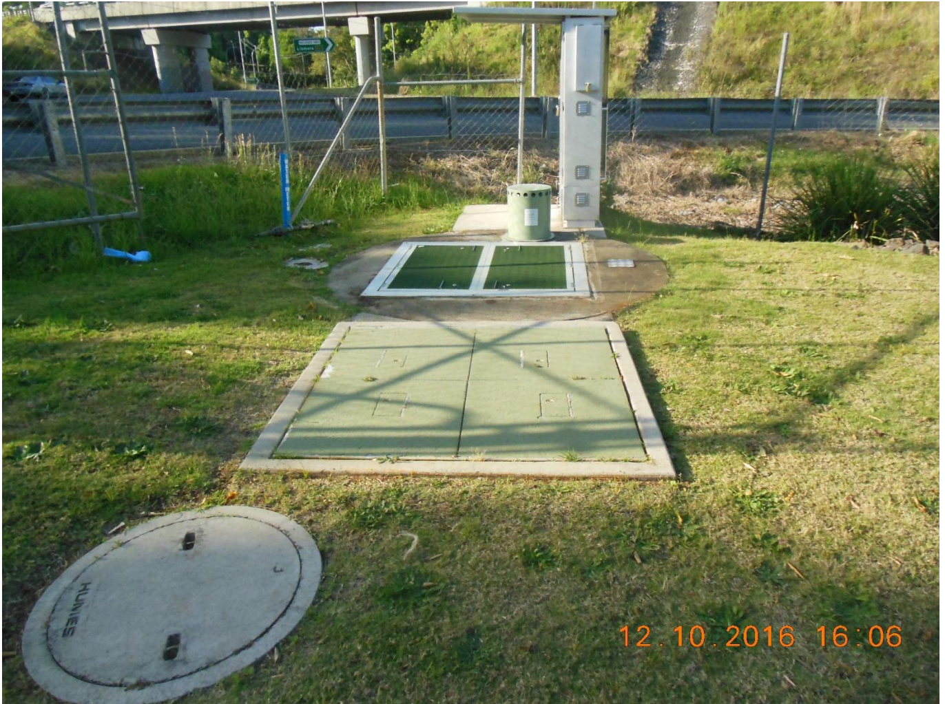
Figure 10 | Council sewage pump station next to westbound off ramp Kays Lane
