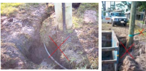
Above: Poles with become unstable if undermined
