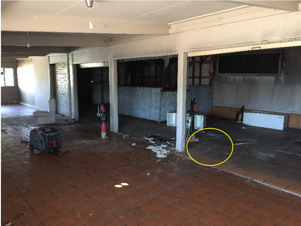
Image 3: Looking west across the front entrance of the building where the location of sample 'S1' is visible next to the concrete corer stand. Fire damage is also visible in the background.
