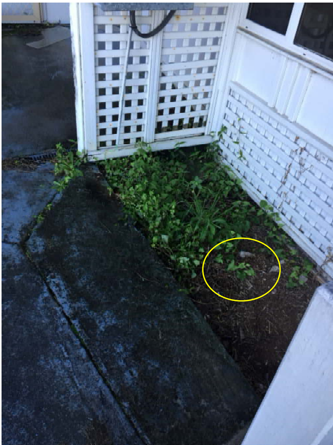
Image 4: A view of the western side of the building where sample 'AS2' was collected.
