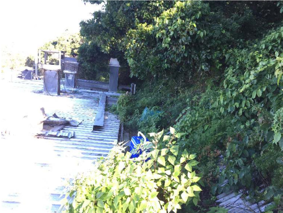
Image 5: A view towards the western boundary along the retaining wall that separates the building and rear yard.
