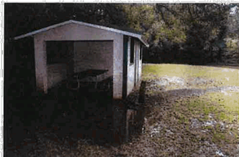
Change Rooms shed after May 2015 flood
