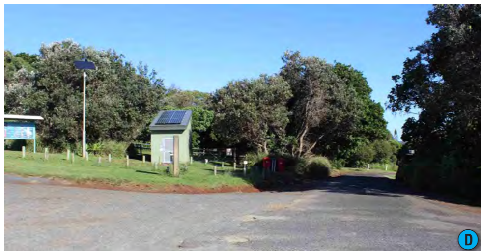
Above: Exit from the car parking area between existing native vegetation. Weathered pavement surface and eroded swale drain.
