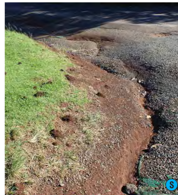
Above: Erosion and water tracking along the edge of the gravel and pavement
