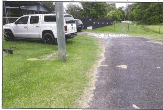
Photo 12 - Existing street hydrants located in Fitzroy Street.
