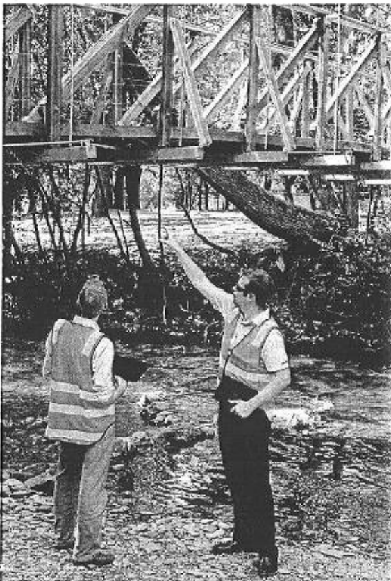
Alpine Council staff inspect a bridge and take notes about its condition using a custom iPad app.
