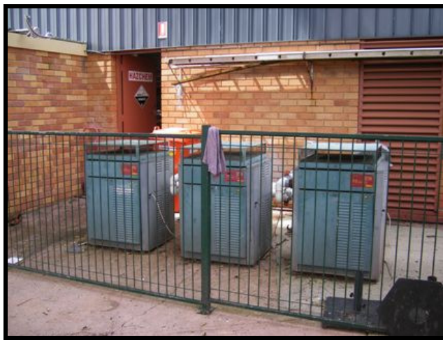
Alstonville Swimming Pool – Existing LPG Pool Water Heaters
