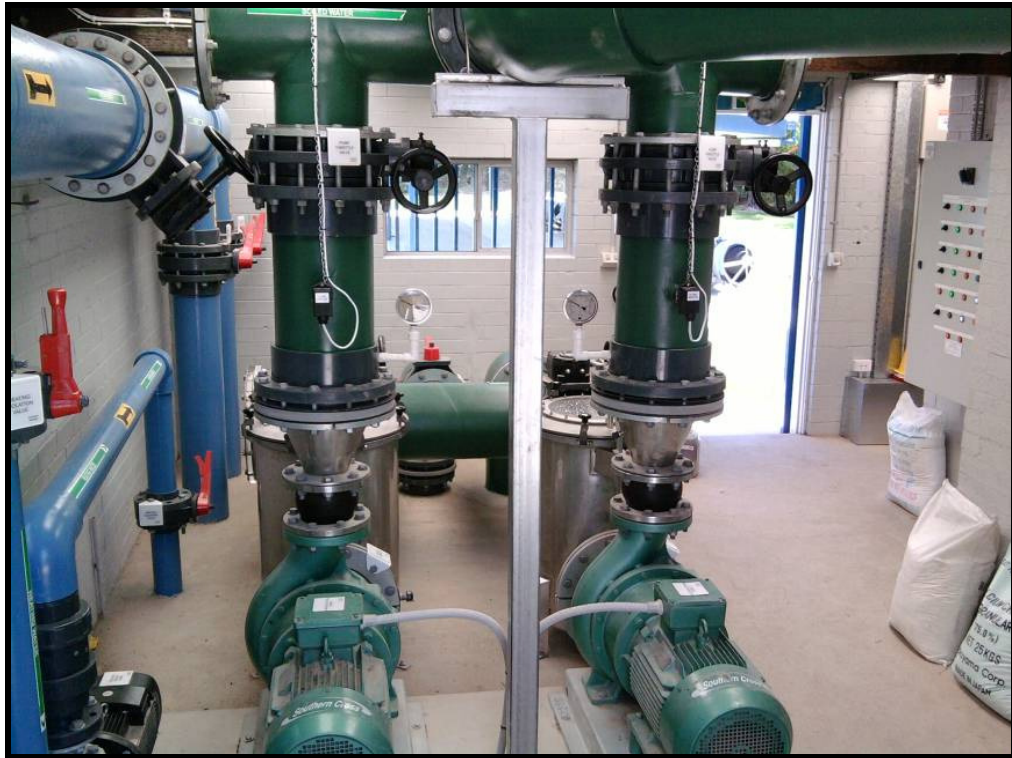
Coffs Harbour Pool Plant Room (November 2010)
