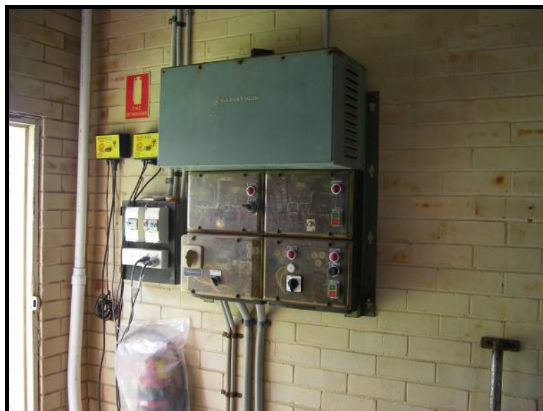
Pool Plant Room Electrical Controls
