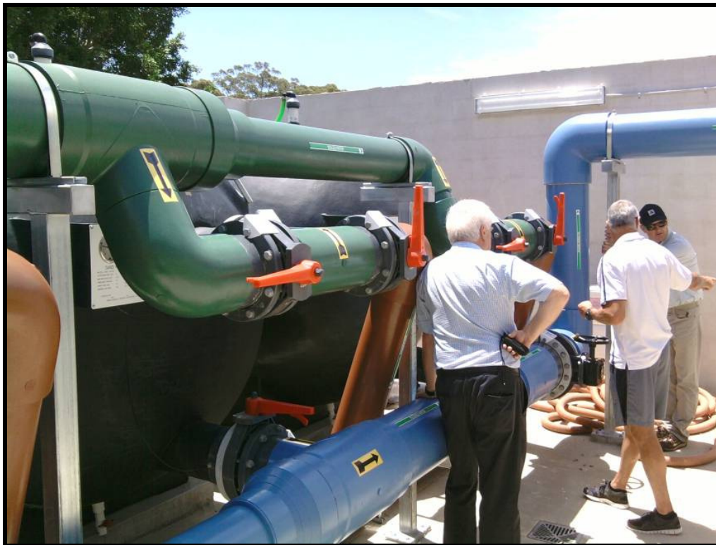
Coffs Harbour Pool Plant Room Filter Area (November 2010)
