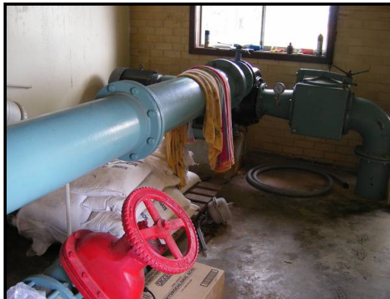
Pool Plant Room
