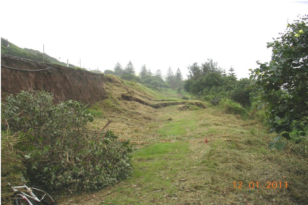
Photo 4: View of landslide head scarp and ground cracks on pedestrian path, looking north west.
