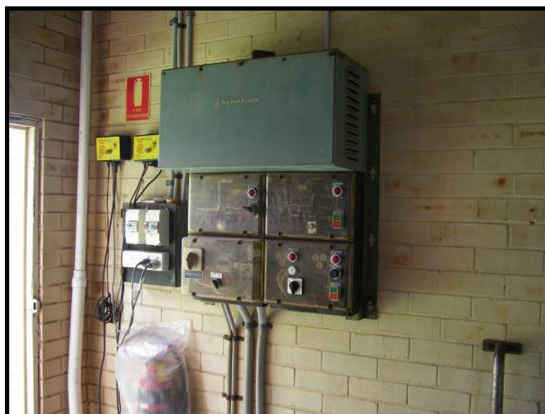
Pool Plant Room Electrical Controls
