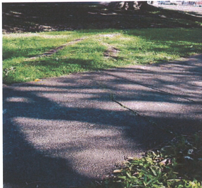
Photo 2: Shows extent of large roots to the north, as well as cracked footpath
