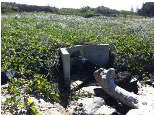
Photo 5: Outlets in inaccessible areas are difficult to access and not regularly maintained (Lennox beach headland)
