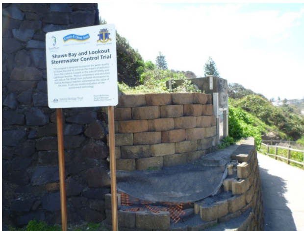
Photo 10: Shaws Bay Stormwater Control Trial
