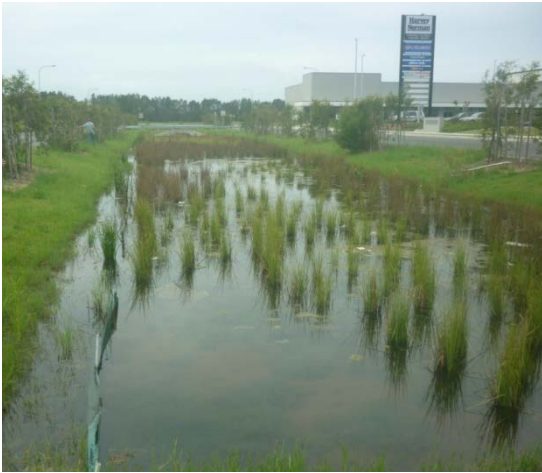
Photo 4: Stormwater drain at Harvey Norman, Southern Cross Industrial Estate. The site does not adequately convey stormwater flows
