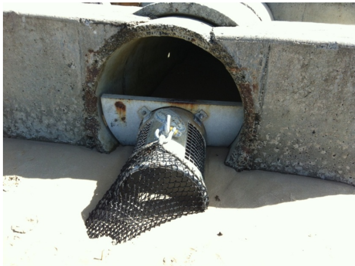
Photo 12: Sock installed on stormwater pipe discharging onto Seven Mile Beach, Lennox Head
