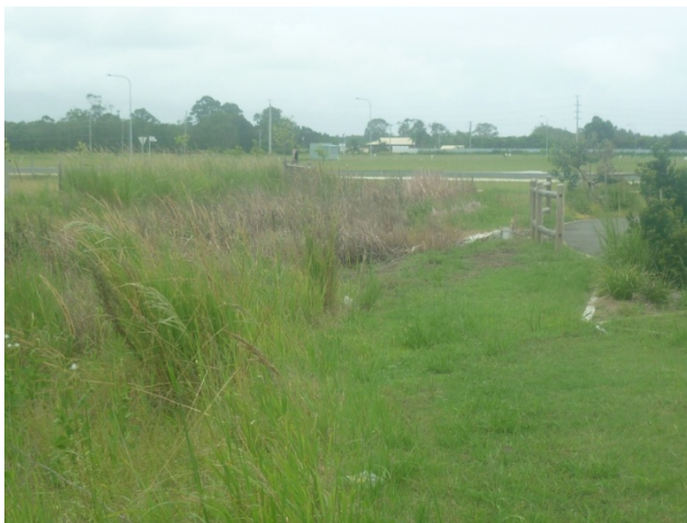
Photo 7: Inadequate maintenance can create blocked drainage (Ferngrove)
