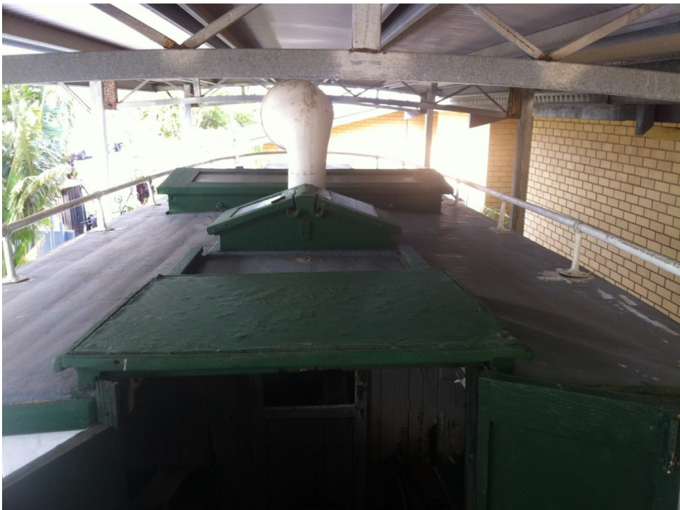
Plate 16: PV Richmond looking across cabin roof. Note intrusive grey fibreglass coating and damage to cabin roof timbers/hatch covers (March 2012).
