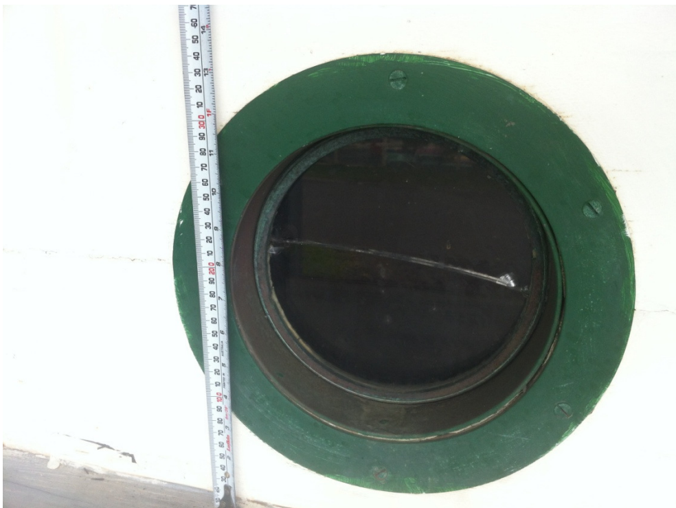
Plate 10: PV Richmond Port Holes; note one port hole/scuttle was missing entirely. The glass in the remaining port holes was all split horizontally. Note corrosion evident under the intrusive paintwork on the brass surrounds.
