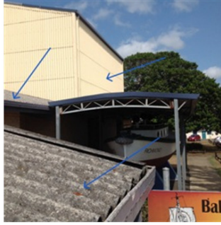
The MV Richmond is Located under metal carport adjacent to acm roof. Friable asbestos is being washed off the adjacent asbestos roof onto the top of the MV Richmond.
