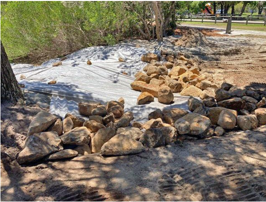
Image: A section of stormwater works as part of the Shaws Bay improvements at Pop Denison Park.
