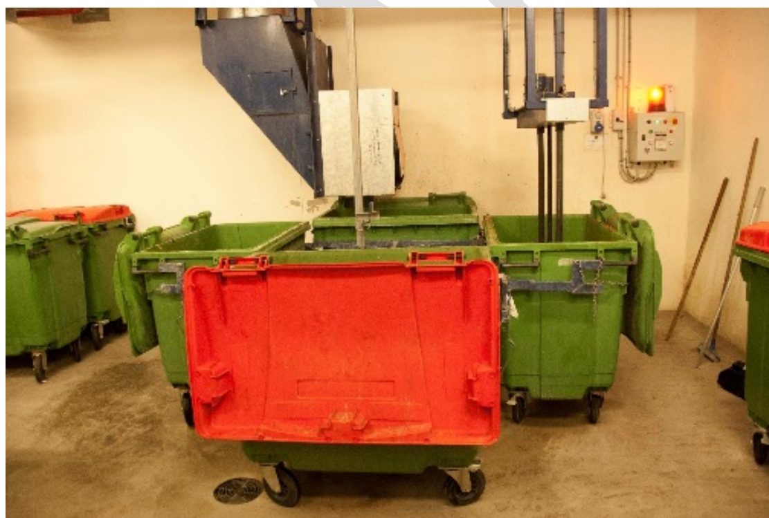
Four x 660L bins underneath a waste chute with a ceiling-mounted compactor with bins rotated manually by the cleaner (Photo: Andrew Quinn)
