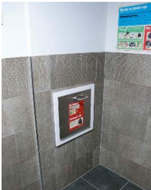
Waste chute inlet located inside a bin storage and service room on each floor of a medium-rise building (Photo: Andrew Quinn)
