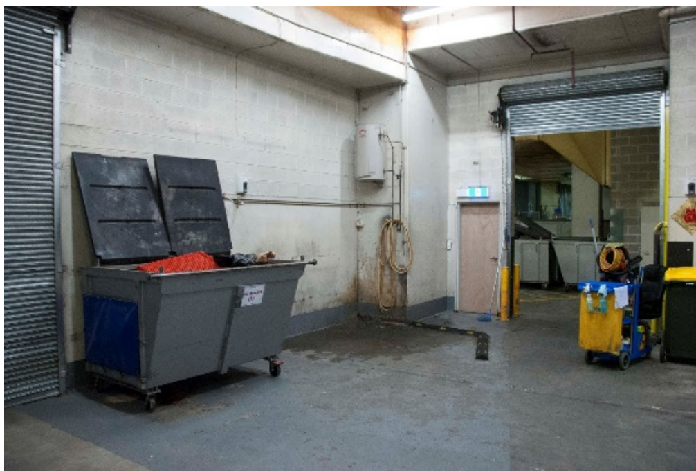
Bin room with an area for cleaning bins, including hot and cold water tap, drain and barrier to prevent water spilling over, and a roller door to access the room (Photo: Andrew Quinn)
