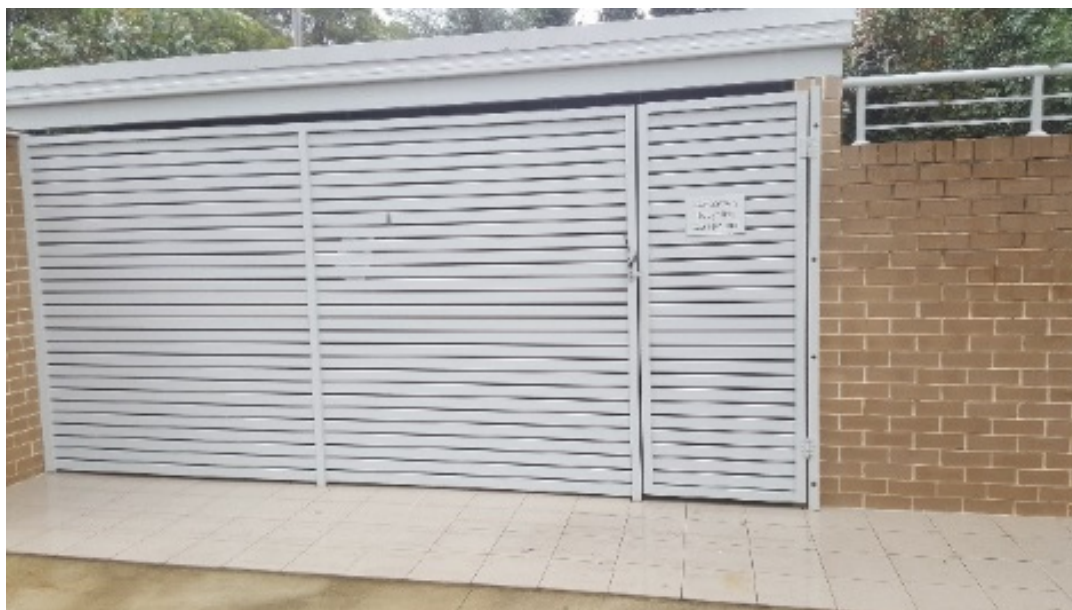
Screened bin storage area fronting a medium-density residential property. (Photo: The Hills Shire Council)
