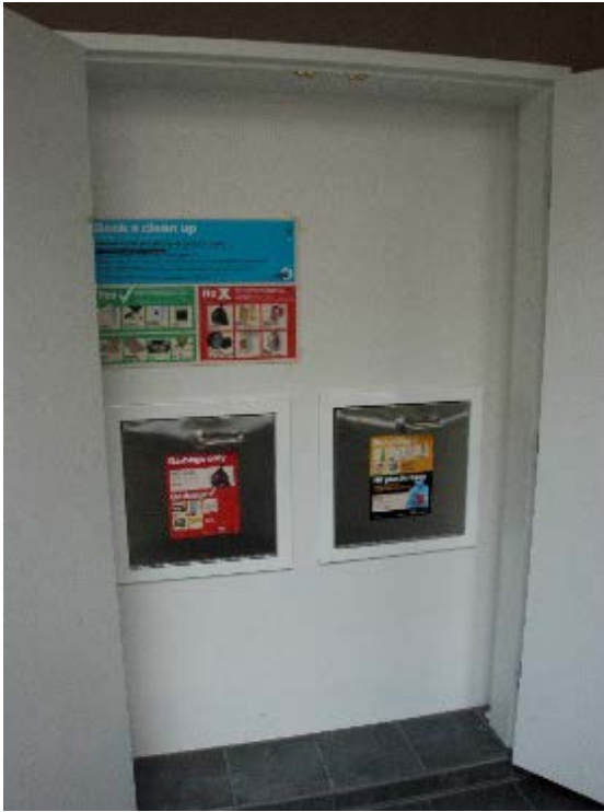
Example of a dual waste and recycling chute inlet in a bin cupboard in a low-rise residential building (Photo: Andrew Quinn)
