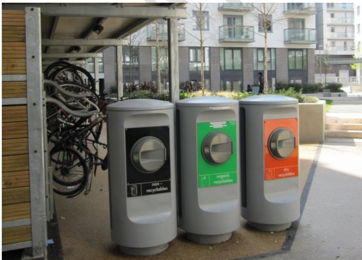
First AWCS installed in Australia (Photo: Sunshine Coast Council) DO we have approval for this photo?
