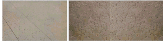
Alternative option - Photographic example of salt finished concrete with regular saw cut joints
