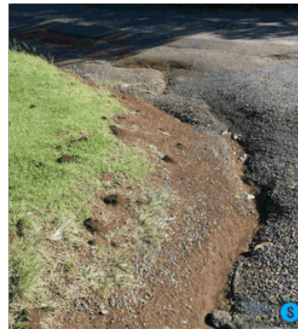
Above: Erosion and water tracking along the edge of the gravel and pavement
