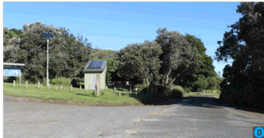
Above: Exit from the carpark area between existing native vegetation. Weathered pavement surface and eroded swale drain.
