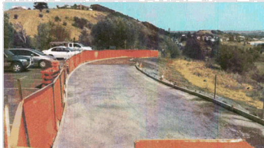
Above: Photograph of pathway construction that was stopped as a result of community opposition
