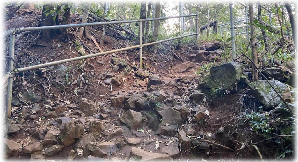
Steel handrail recently installed on steep section of path down to creek
