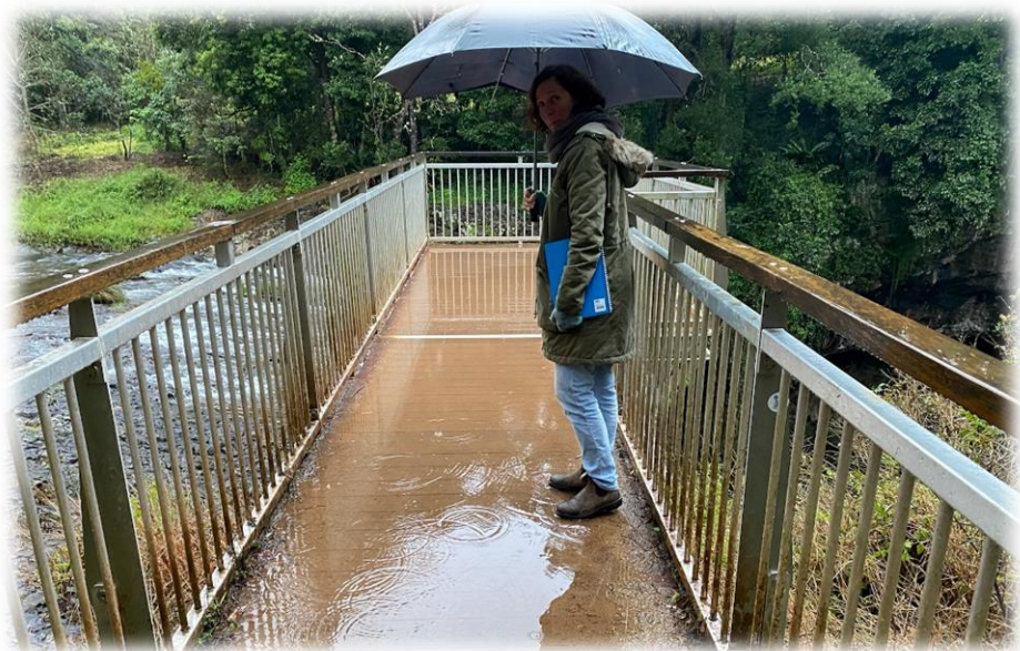
Pooling on the lookout platform
