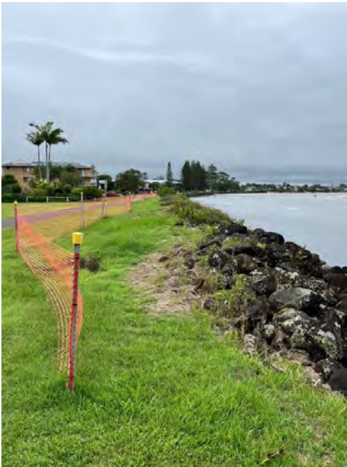
Figure 13: View looking northwest at Site 2.4 located within Lot 7036 DP 1068936, Crown Land managed by BSC (Namatjira Place Foreshore Reserve); USL within North Creek for land above and below HWM; and, Commemoration Park Lot 7006 DP 1068885.
