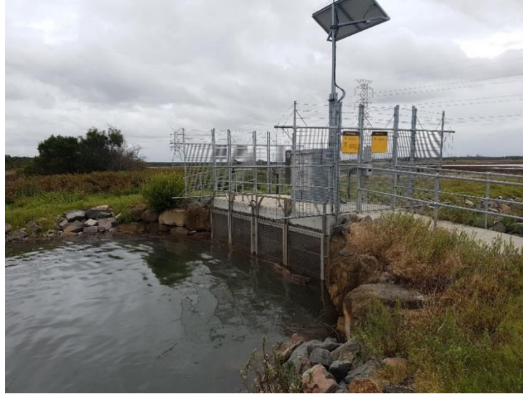
Figure 3.1: Example of automatic gates controlled by water level gauges (Kooragang Island, Hunter River)
