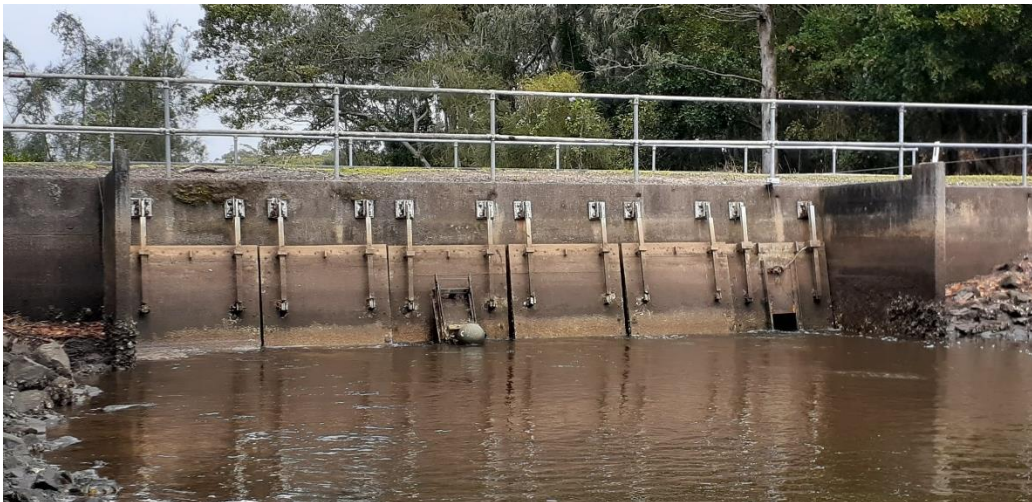
Figure 3.2: Sluice gate (right) and buoyancy driven tidal gate (left) on the Keith Hall floodgates
