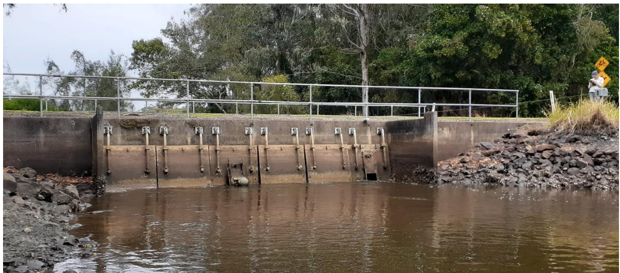
Figure 2.10: Keith Hall floodgates (October 2020)
