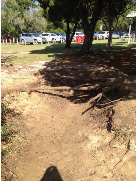
Photo 3: Erosion to be remediated by beach nourishment at Middle Pop Denison Park Beach
