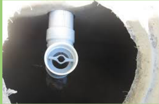
Figure 3: Position of septic tank outlet filter inside PVC pipe – outlet tee junction
