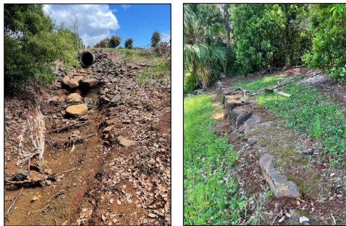
Plate 30: The stormwater channel from Elvery Lane requires rock lining (left) and the northern bank area (right).
