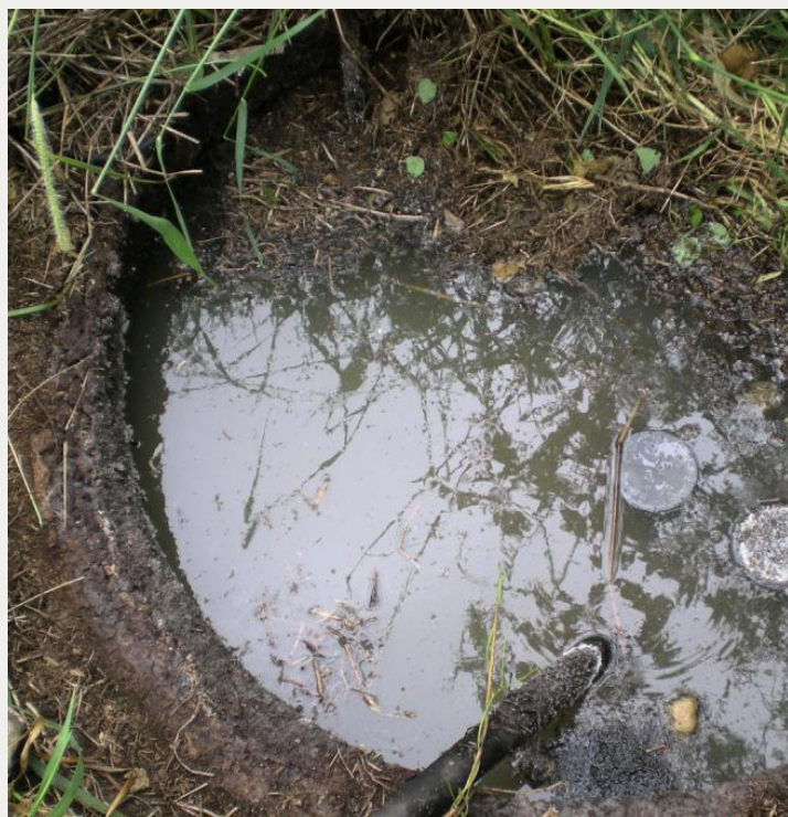
Aerated Wastewater Treatment System – flooded and no power supply to pumps.
