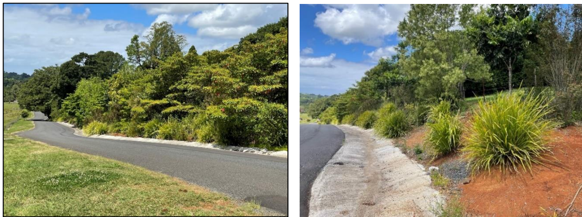
Plate 35: Some bare patches occur around Lomandras, apparently eroded during flood rain (left), and stormwater channel (right).
