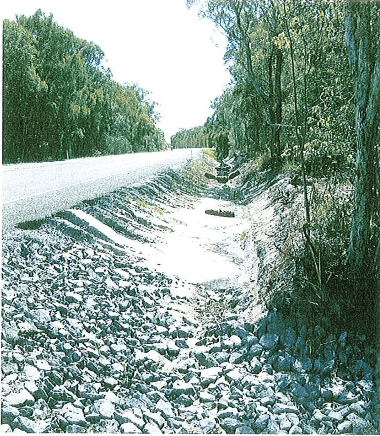
photo 4: Recent road works and bare soil channel
